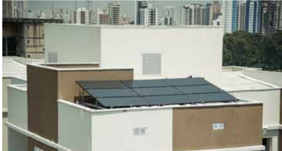
Allegro Jardim Avelino Building, in São Paulo (SP) - Solar panels
